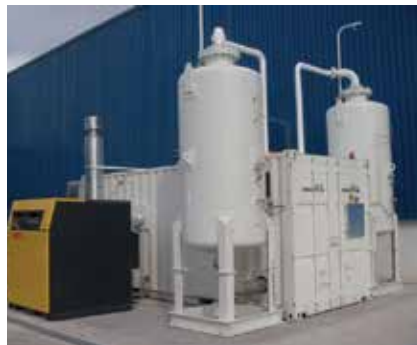
Halia Modular Aeration System
