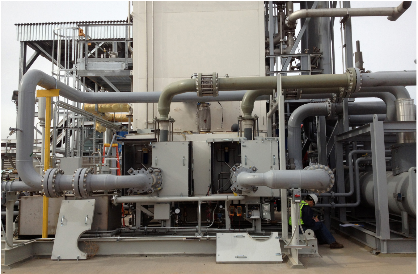
Commissioning of an Air Products compander pair at a plant in Chandler, Arizona
