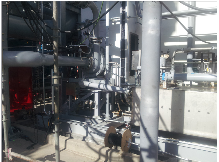
Air Products compander installed at a plant in Miami, Arizona
