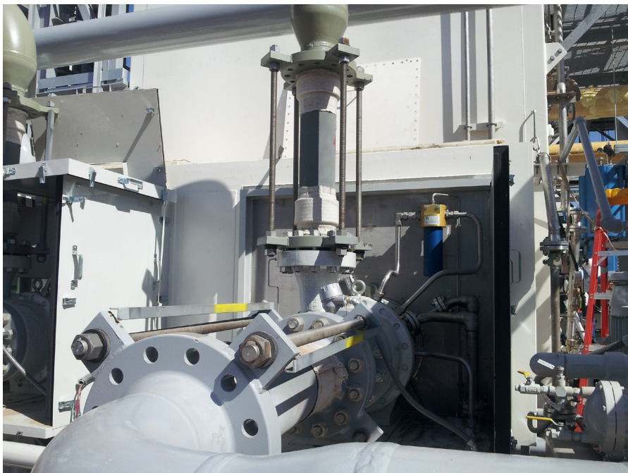
Air Products compander installed at a plant in Chandler, Arizona
